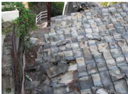
4-(1)-① 剥落又は脱落
