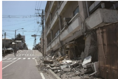
Building with its first floor collapsed due to the fierce earthquake
