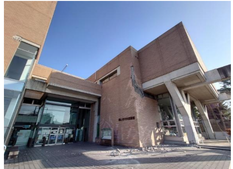
Koriyama Municipal Chuo Library where a wall collapsed
